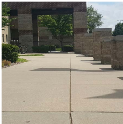
Image 24: Excessive Cross Slope in Walk
